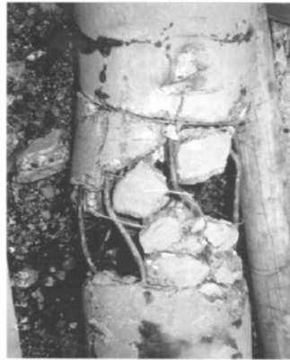
Fig.2. Damage to pile by 2m of lateral ground displacement during 1964 Niigata earthquake (Yoshida et al. 1990).
