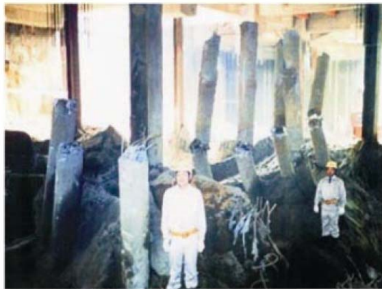
Figure 3. Excavated piles of a building twenty years after the 1964 Niigata earthquake. The superstructure is three-storey RC building. The piles are precast RC piles 10 m long and 300 mm in diameter. (Photo courtesy: T. Tazon.)
